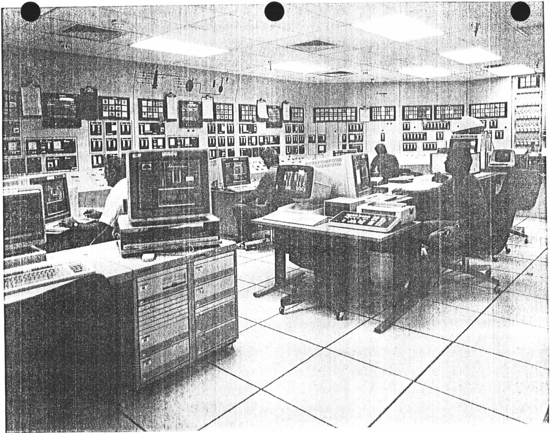
FAST MAIN CONTROL ROOM
