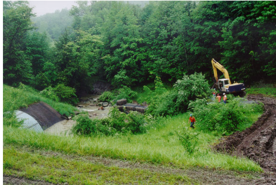
Work on the 1.8 mile rail spur at the WVDP was one of many preparations at both the WVDP and INEEL.
