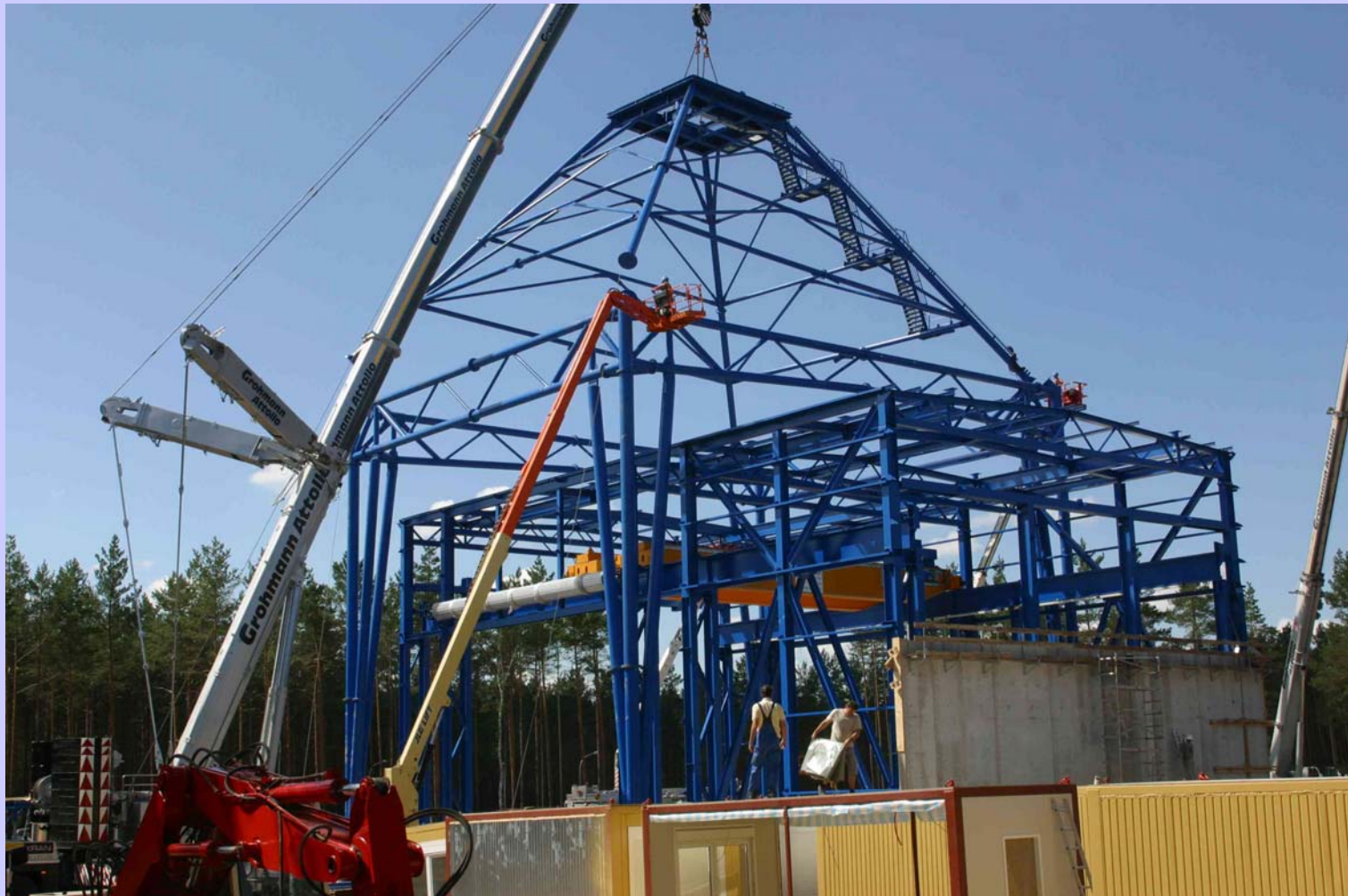
Top of drop tower being hoisted into place by an 80-ton portable crane.
