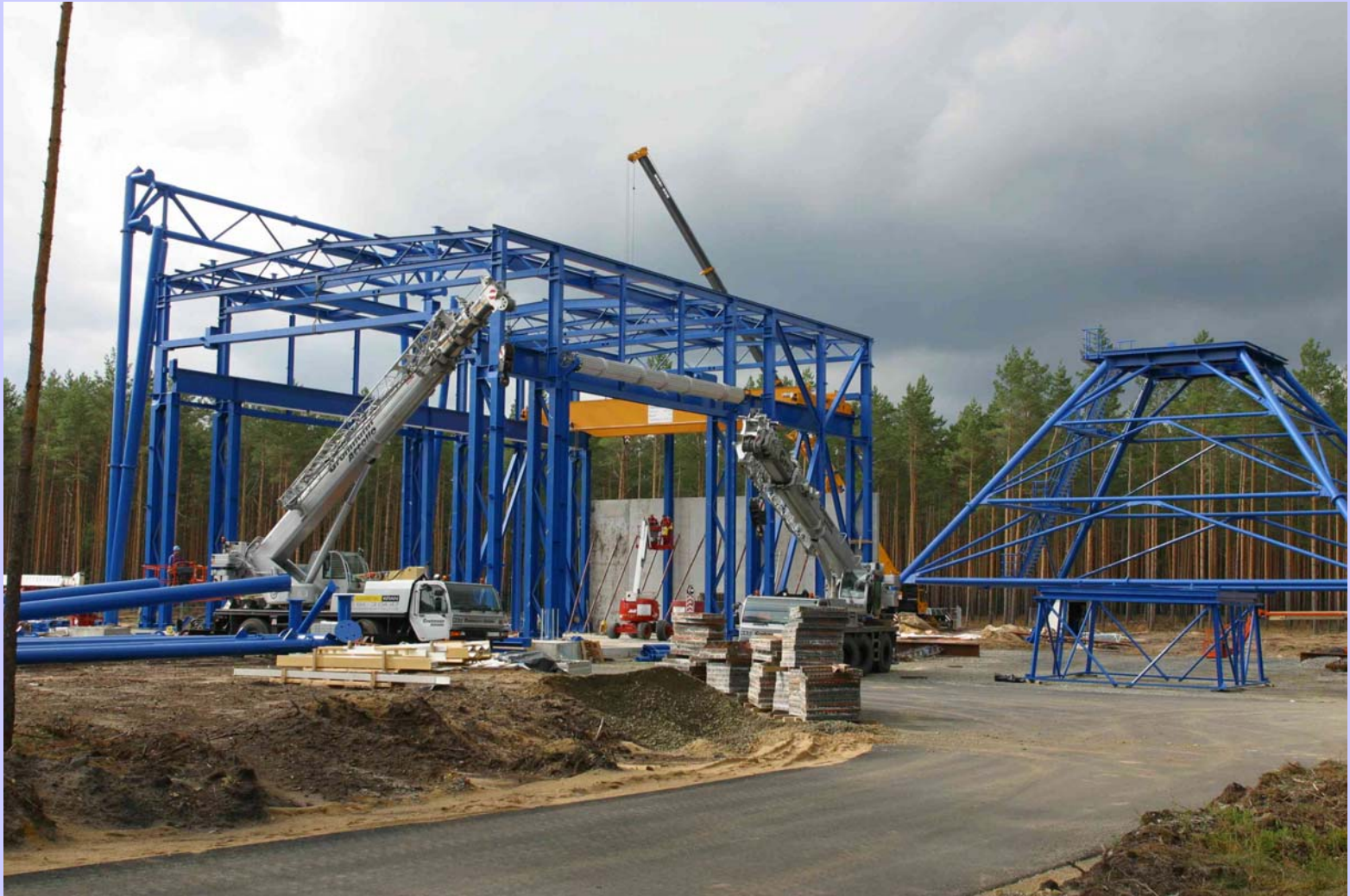
Finished skeleton of enclosed test building (left) and top of drop tower (right)
