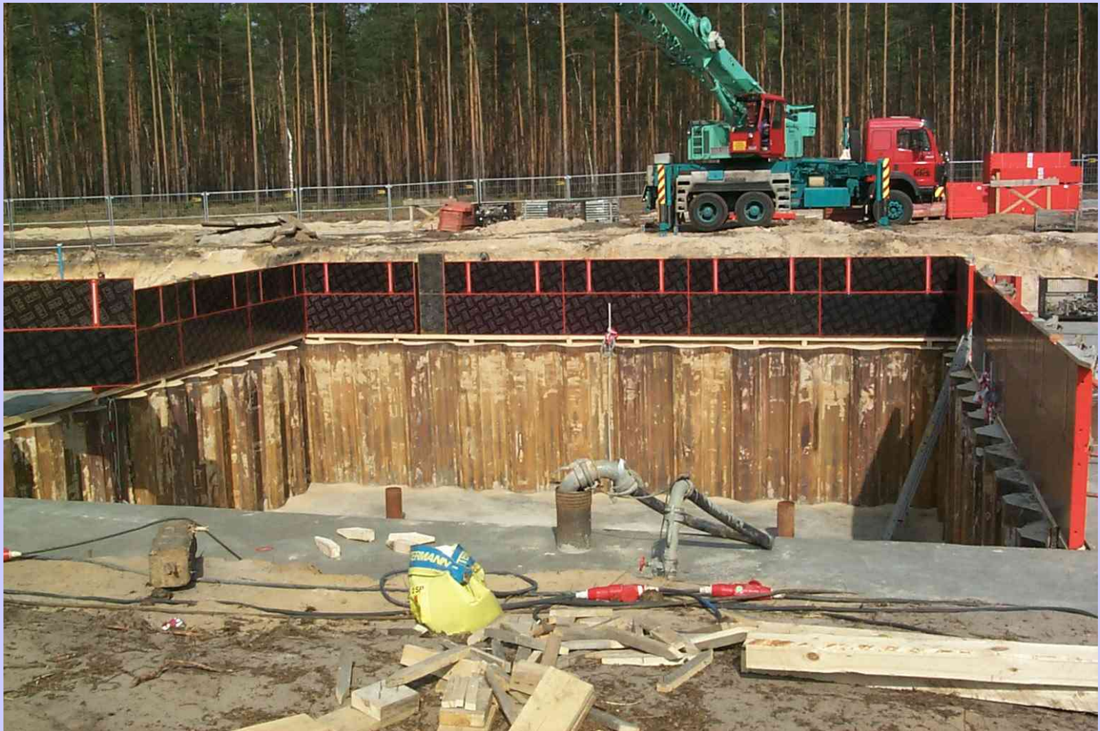
Excavation and lining of a cavity for the unyielding surface . (46 ft x 46ft x 16.5 ft).
