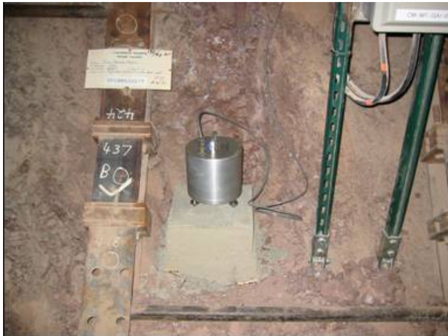
Underground Strong-Motion Seismic Monitoring Station
