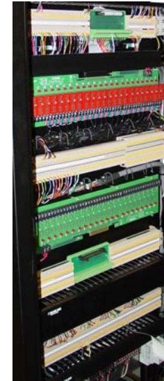
Interior of control cabinet
