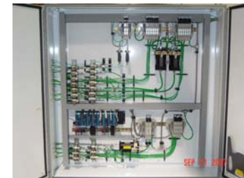
Utility control system (instrument air, helium, and argon/helium mixture)
