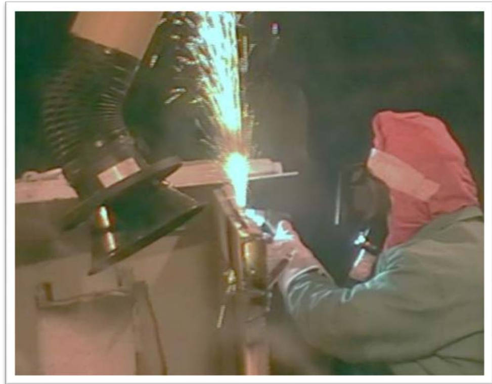
Using plasma cutting to process the first plutonium contaminated TRU waste box in the CSRF
