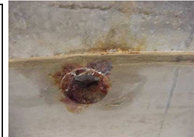
Cask bottom cover plate bolt corrosion observed in 15-yr demo at INL
