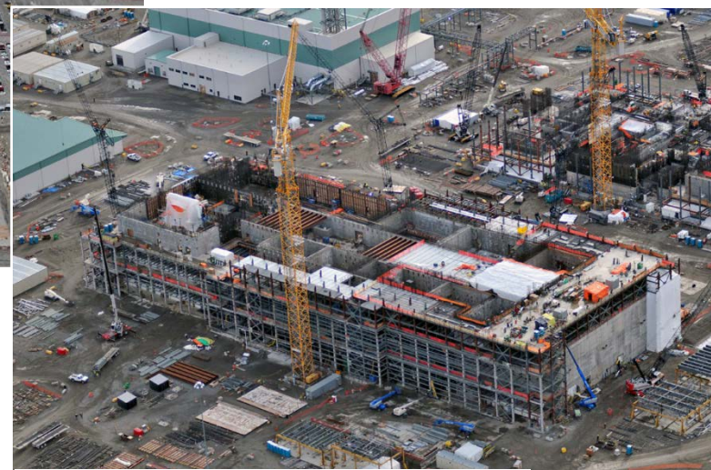
Pretreatment Facility (PT)
