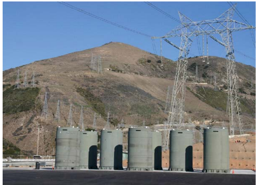
Dry cask storage at Diablo Canyon
