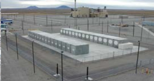
TMI – Horizontal modular dry storage
