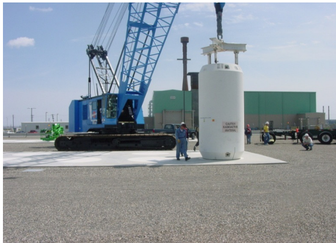
Dry Cask Storage
