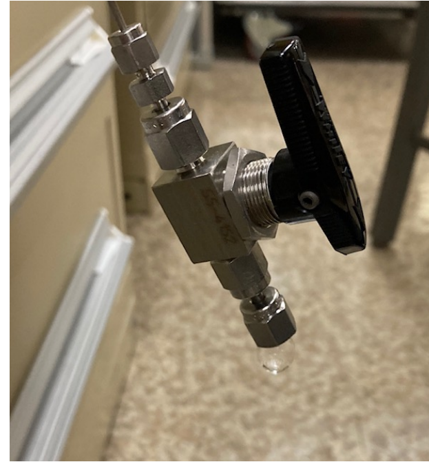
Visible water release through sampling line during heating
