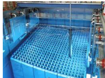
Spent Fuel pool
