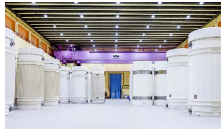
Dry Interim Storage
