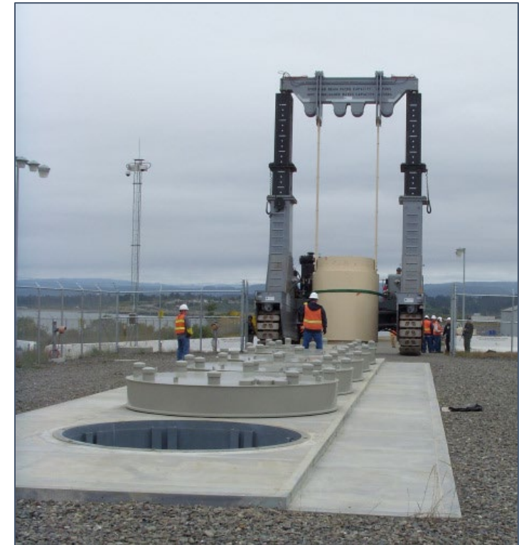
Photo from Holtec International
