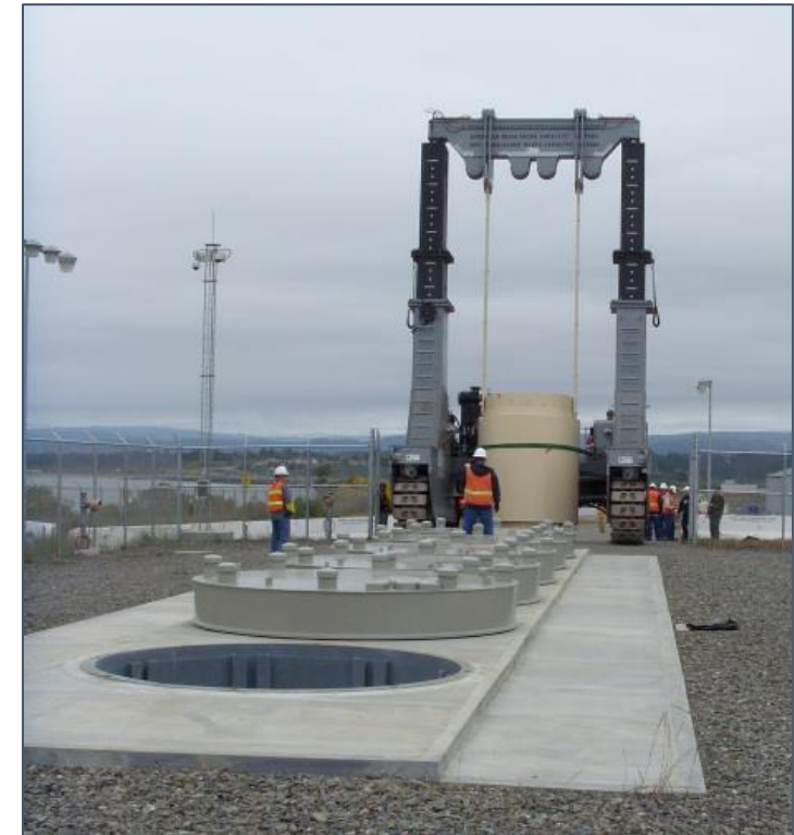
Photo from Holtec International
