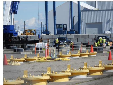
CPP-749 Underground Dry Storage
